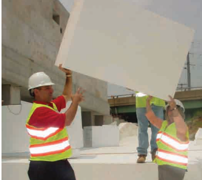
Joyce Curtis (right), director of the FHWA Resource Center, assists in a product demonstration of expanded polystyrene (EPS) geofoam on the Woodrow Wilson Bridge project in northern Virginia. EPS geofoam is a rigid foam plastic engineered with a unit density as low as 1 pound per square foot, making it a lightweight fill that is 100 times lighter than most soils and useful on some transportation projects.
