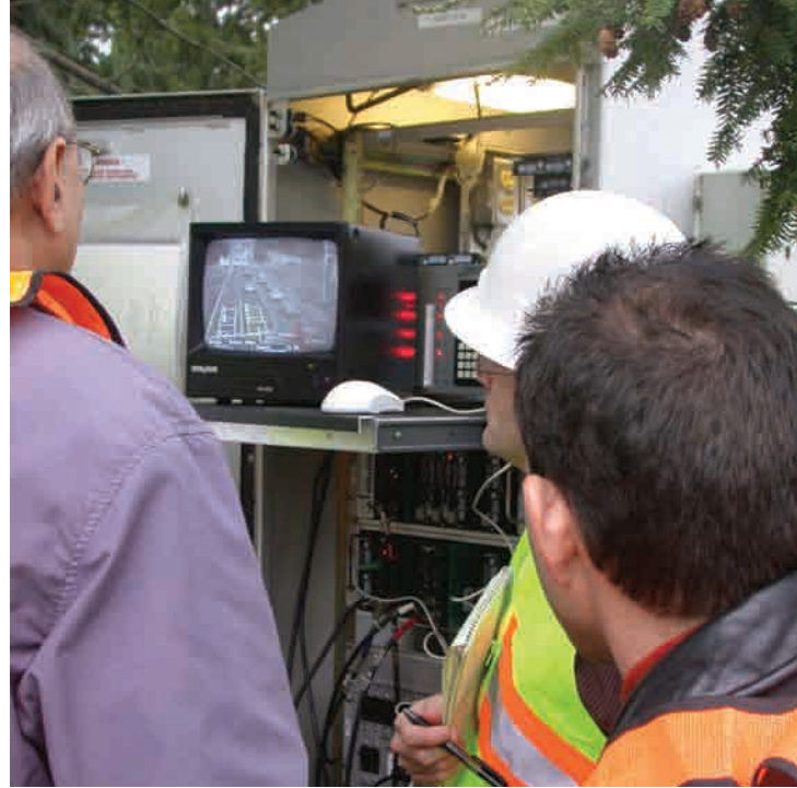
Personnel from FHWA and the Virginia Department of Transportation calibrate a video image processor, a type of over-roadway sensor, one of the many forms of ITS technologies that can be integrated into a transportation system to smooth traffic flow.
