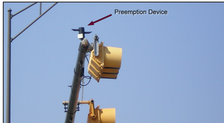
Photo by: Texas Transportation Institute
