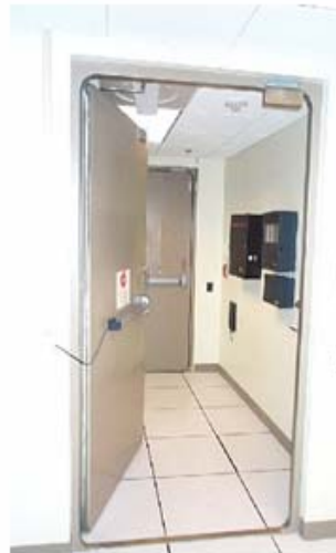
Man Traps secure entrances into sensitive Data Center areas
