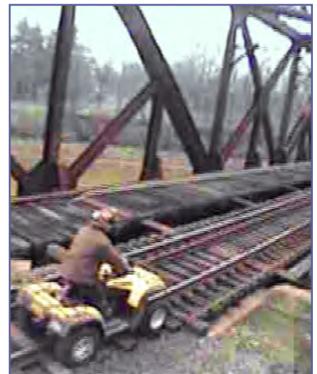
Railroad Bridge Security: Video image of a trespasser on a railroad bridge.
