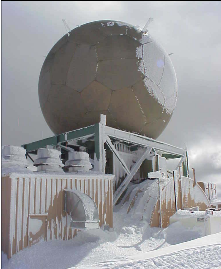
Figure 3: Missoula WFO Radar at the top of Point Six
