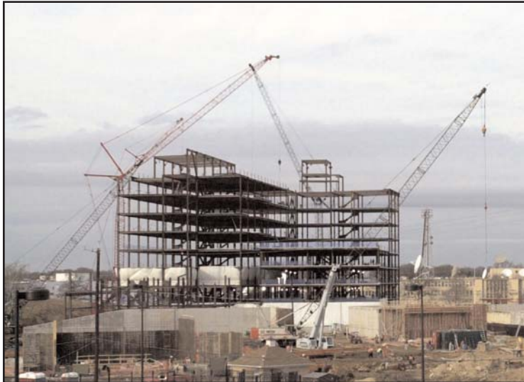
Photo by Richard Reed for U.S. Census Bureau. The new Census Bureau building, scheduled for completion in late 2006, is part of a complex under construction in Suitland, Maryland.
