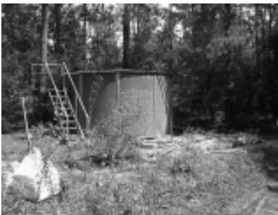
Tank at Dominican Republic spill site
