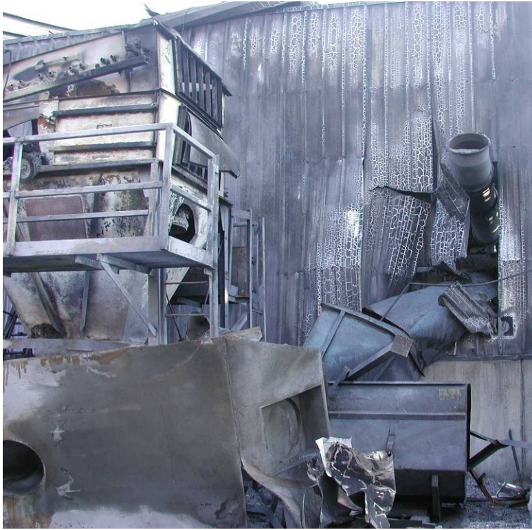
Figure 14. Hayes Lemmerz did not follow NFPA 484 guidance on locating and maintaining the dust collector, which exploded on October 29, 2003.
