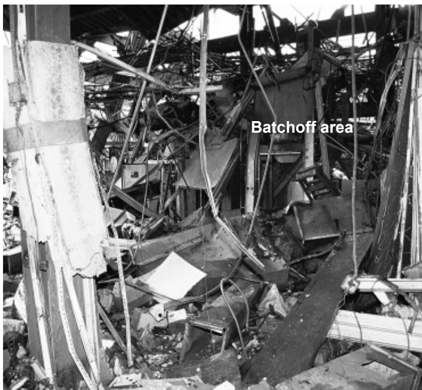
Figure 11. Extensive damage and debris near mill and batchoff machine #1.
