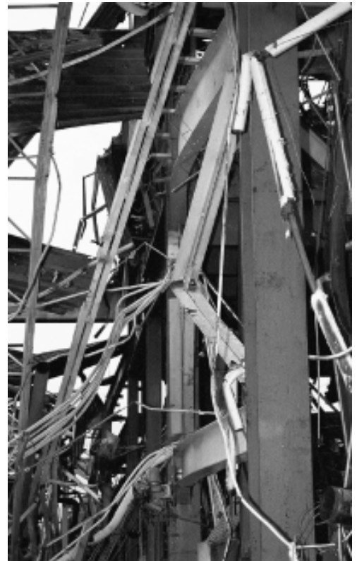
Figure B-1. Beam and cross bracing deflected southeastward toward warehouse.
