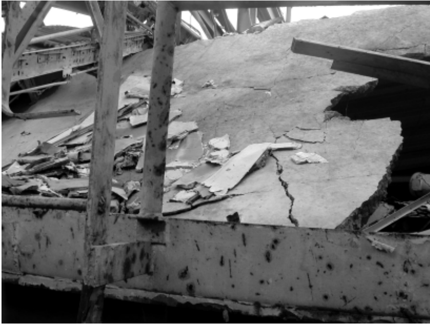
Figure B-2. Uplifted concrete floor in mixer area.
