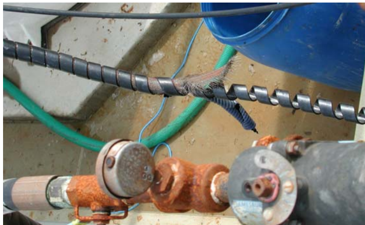
Figure 2. Failed stainless-steel transfer hose.
