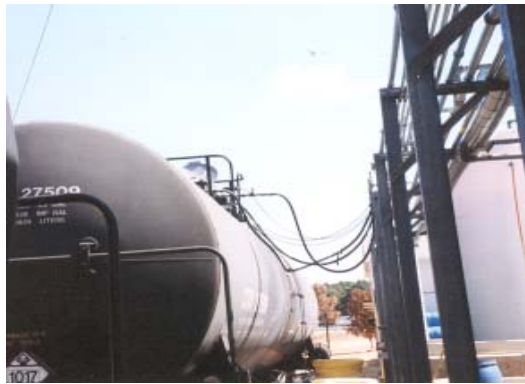
Figure 1. Railroad tank car unloading station #3.
