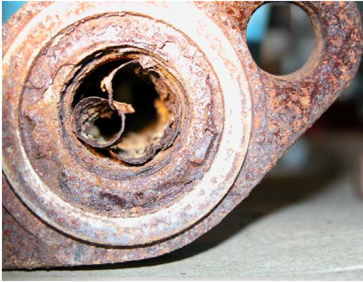
Figure 25. Corrosion buildup in chlorine repackaging piping system.
