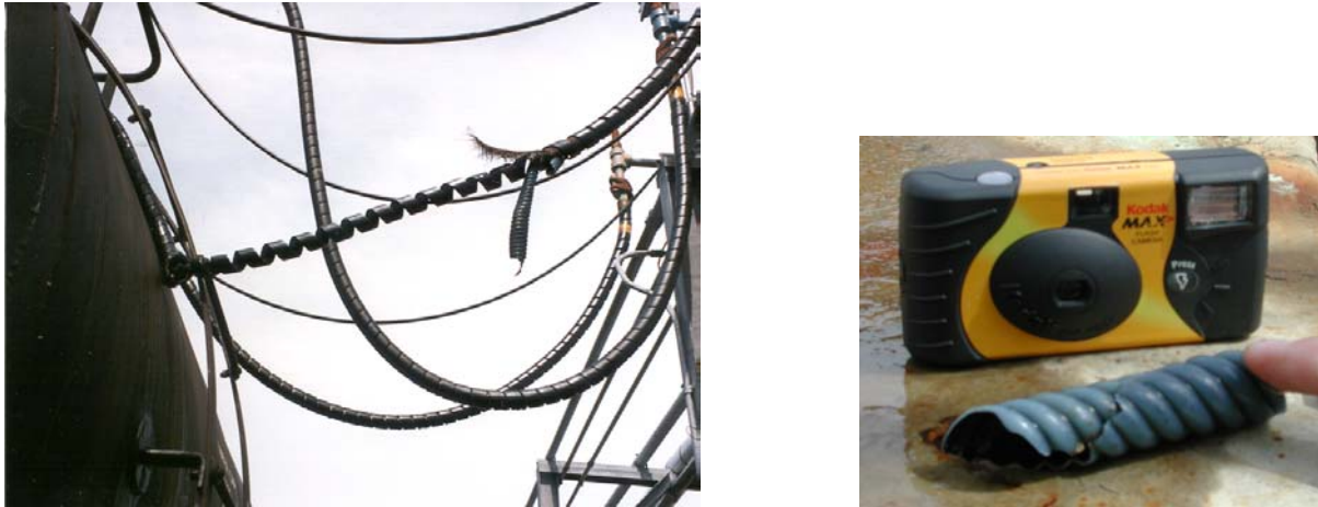
Figure 21. Ruptured hose and piece of Teflon inner liner.
