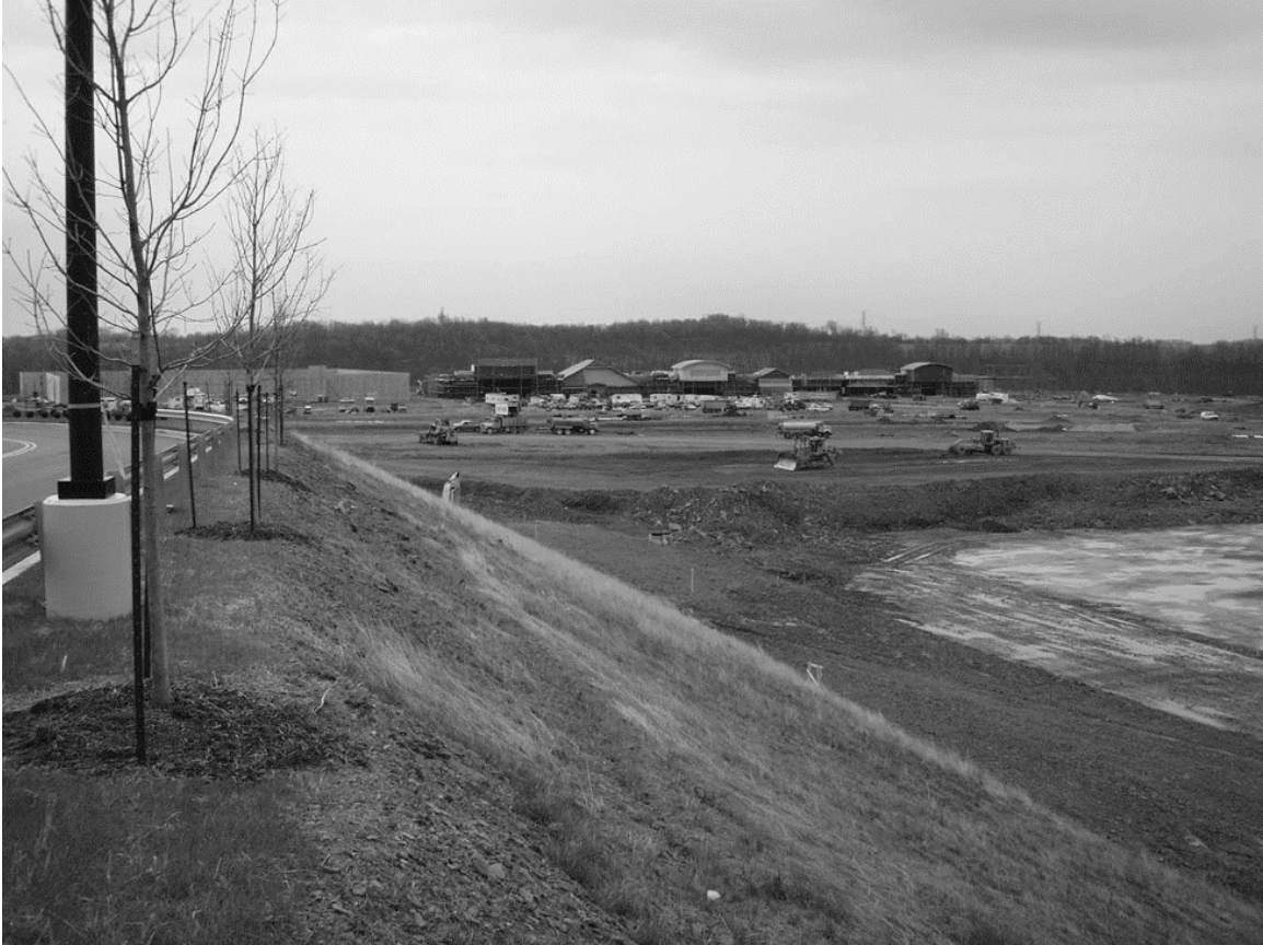
Figure 4. View of a small area of the Highlands Complex that is being built partially on a mine refuse dump. The buildings in the background are not located on the mine refuse fill. The area in the foreground is located over part of the refuse dump that has been subsequently filled with material from the current site preparation. During a recent site visit we observed new construction taking place on this filled area.
