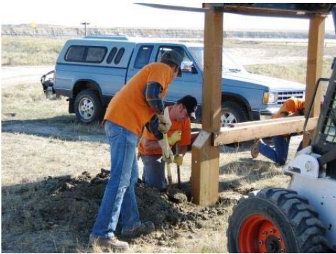
National Public Lands Day volunteers tamp dirt and position an interpretive kiosk as part of several work projects conducted Sept. 30 on BLM-managed land northwest of Terry. Volunteers installed a gate, performed trail maintenance and hauled away refuse during the 13 th annual nation-wide event.
