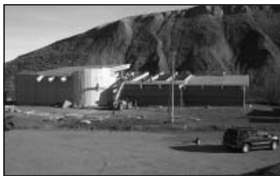
Workers install roof panels on the new interpretive center in Fort Benton. Photo by Connie Jacobs.
