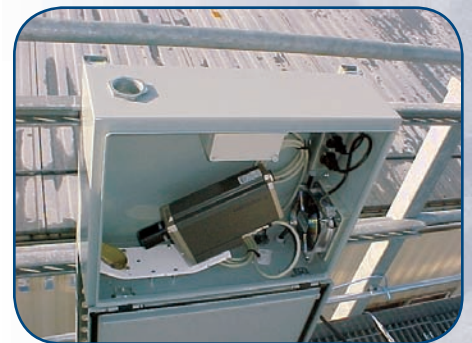
A filtered fan keeps moisture from building up on the mirror surface (bottom left) by circulating air up through the optical port (top left) of the IRT enclosure.
