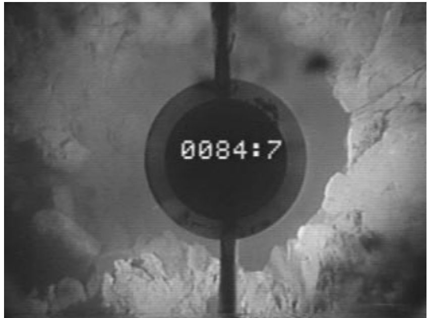
Figure 14. Image from borehole television survey showing fracture at 84.7 feet below land surface in well CC-7, Malvern TCE Site, Chester County, Pennsylvania.
