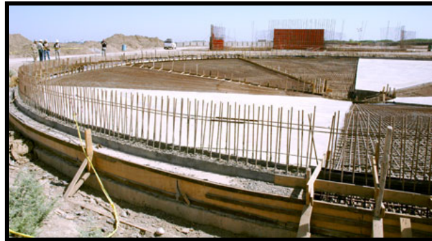
Figure 3.2: Clarifier Tank in Erbil, Iraq
