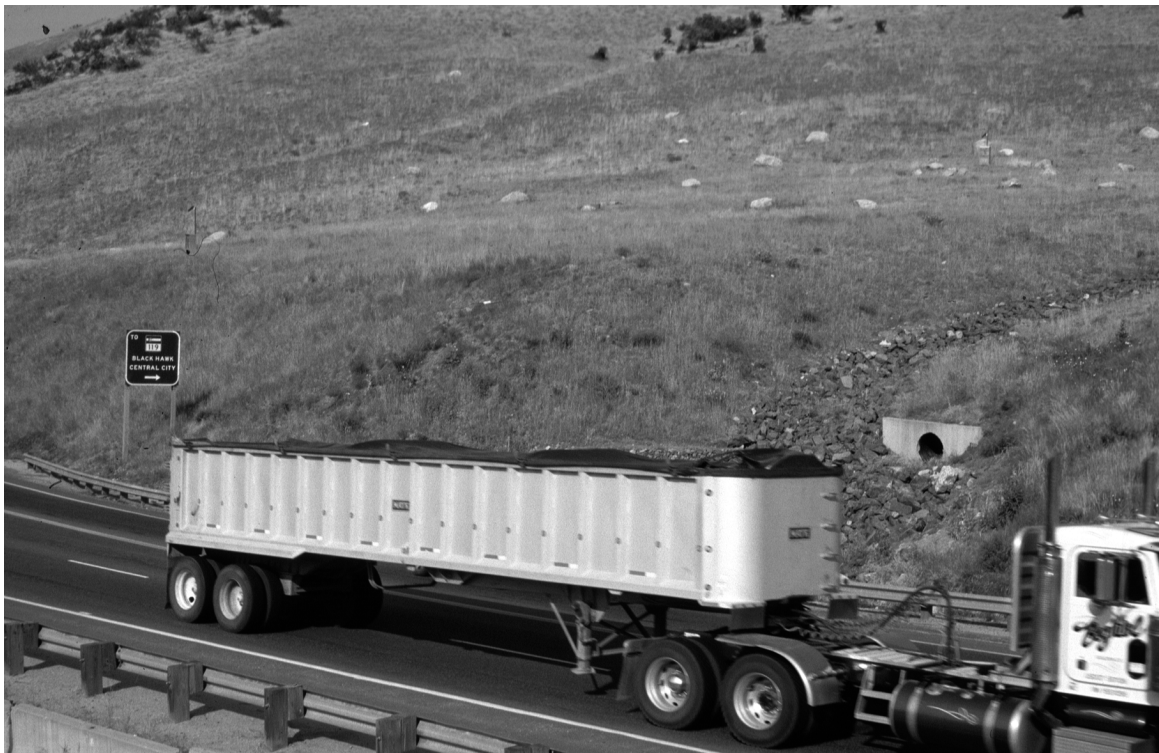
Fig. 26. Environmentally-friendly stabilization of a cut slope on Colorado State Highway 93 in Golden, Colorado, U.S.A. (A) Installation of 3m x 3m reinforced-concrete “face plates” tied to a system of rock anchors (photo: March 1994). The final rock-anchor system consisted of three rows of anchors with a total of 40 anchors and face plates. (B) Post-construction view of same site (photo: July 2003). Anchors and plates have been hidden by a soil fill, which has been planted with native grass.
