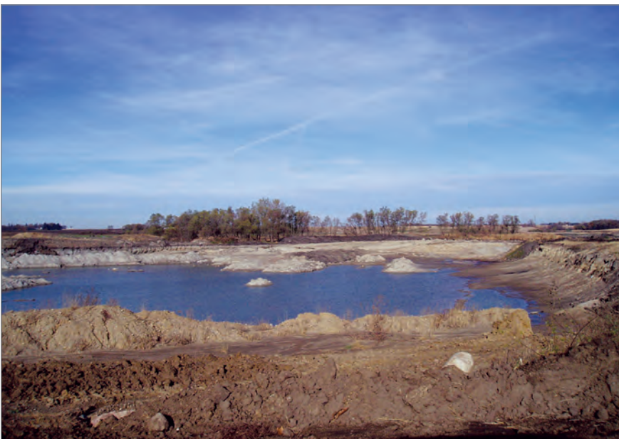
Figure 13. Lands in transition from one land use category to another pose unique challenges for image analysts. Field inspection of this site indicated the area was under construction as part of a highway project.
