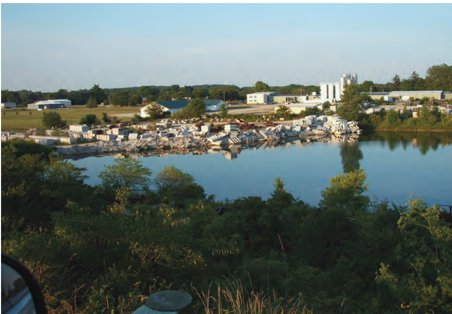
Figure 44. Examples of wetland loss. Fill being placed into a wetland pond in Ohio, 2005.
