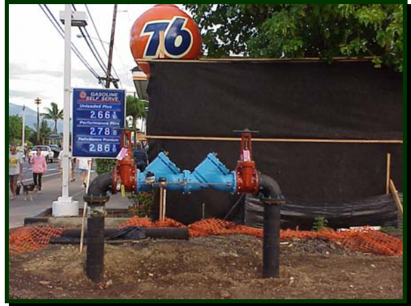
With development come infrastructure issues that have environmental implications, such as pipelines, above.
