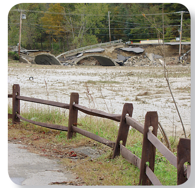
This bridge over the Cold River collapsed during the October 9, 2005, flooding in Walpole, NH.
