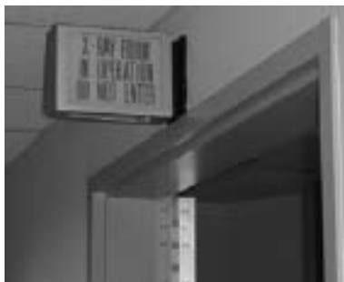
Figure 5.51. The door interlock prevents unwanted exposures; the lighted sign provides additional mistake-proofing.
