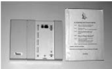
Figure 5.70. This system uses an audible alarm; posted instructions aid in troubleshooting.
