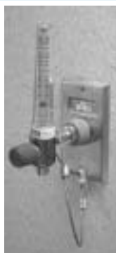
Figure 5.12. A regulator attached to the wall with steel cable.
