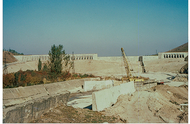
Figure 32. Photograph of construction of a cellular reinforced-concrete debris-retention dam on the Bolshaya Alma-Atinka River of Kazakhstan. This 40-m-high dam, which was built in 1981–82 to protect the city of Almaty from the many debris flows from the Tien Shan Range, is founded on debris-flow deposits. Photograph taken in 1981 by D.J. Varnes, U.S. Geological Survey.
