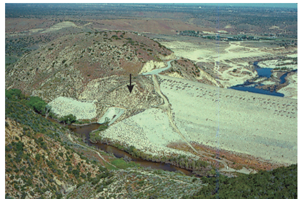
Figure 40. Oblique view of the left end of Mojave River Dam, an earthfill flood-control structure in southern California, United States, showing the two earth berms that were added to the left abutment to buttress a small abutment slide (marked by arrow) that occurred during construction. Photograph taken in 1998.
