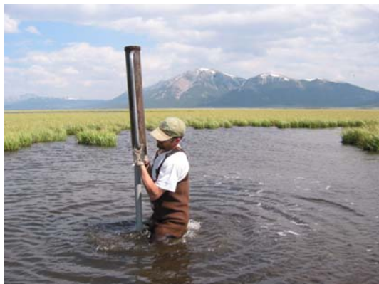
A researcher installs a monitoring well at Red Rock Lakes National Wildlife Refuge.
