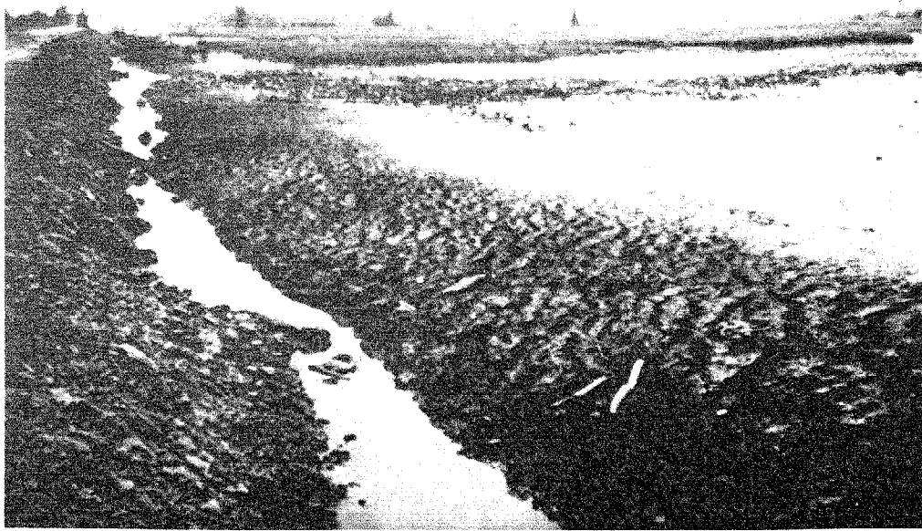
Figure 30. Marsh deposits at Magee Marsh, showing tension cracks that develop when dewatered (Savoy 1956).
