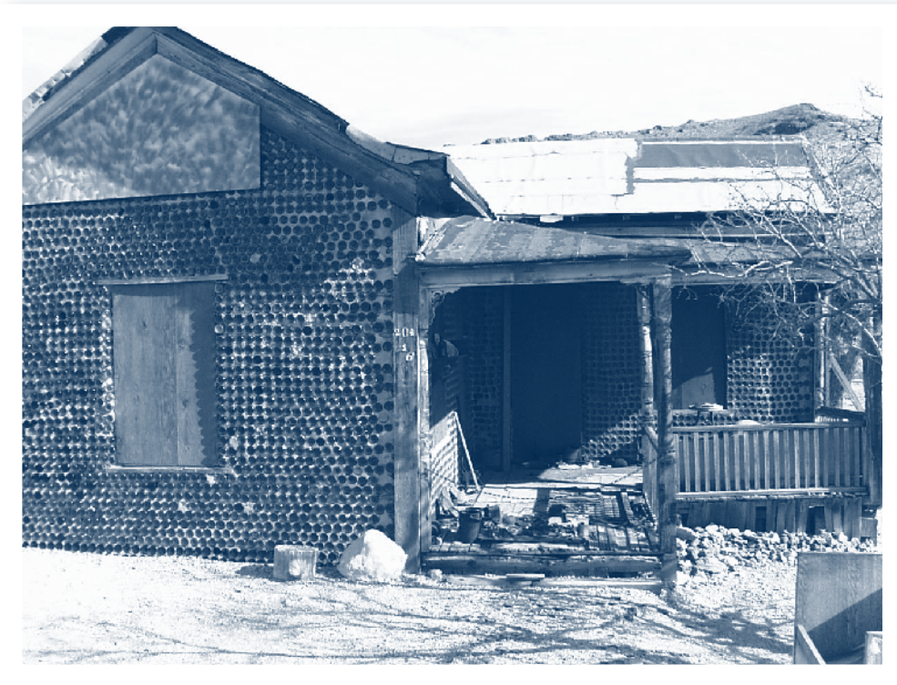
RHYOLITE BOTTLE HOUSE BEFORE THE REPAIRS.
