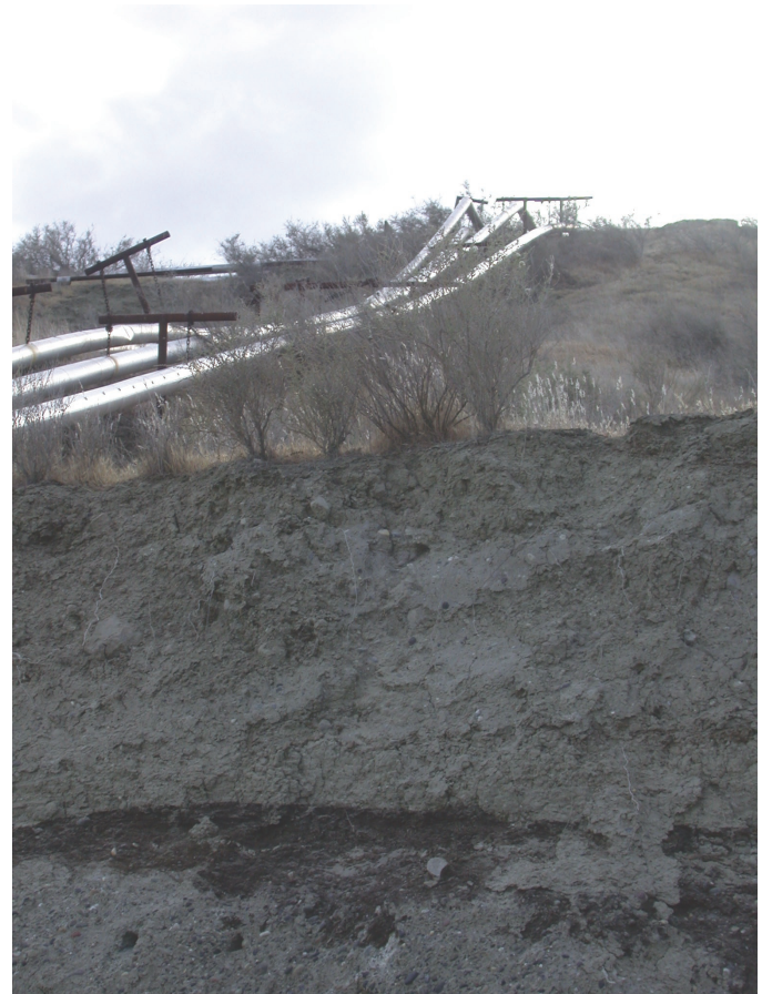
Figure 3.57. Lines route steam where needed in this oil field near Coalinga, California.
