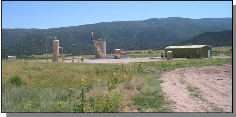
Figure 9. Typical Compressor Site
