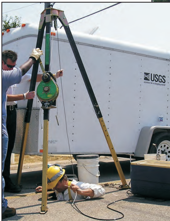
USGS and MWRDGC personnel making a confined-space entry for installation of an acoustic sewer flowmeter.
