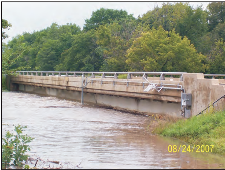
Downstream side of the U.S. Route 6 bridge on Aux Sable Creek, Grundy County.
