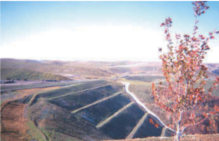
Figure 16. Photograph showing view of excess-spoil fill, or valley fill, in the Samples Mine, Boone and Kanawha Counties, W. Va. The valley fill is stabilized, terraced, and seeded. Photograph by Susan J. Tewalt.
