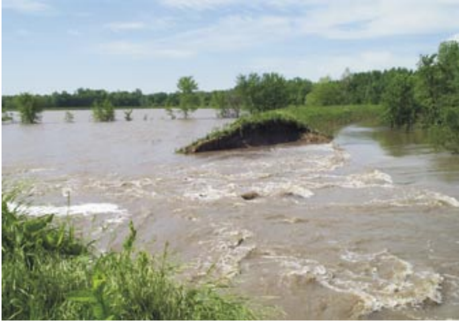
Levee breaches were a common occurrence during the Great Flood of 1993. More than 1,000 Federal and non-Federal levees were topped or failed during the flood. Photo by Perry Draper, USGS.
