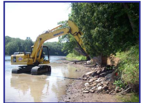
-USFWS An excavator stabilizes the bank along the Menominee River in Marinette County, Michigan.
