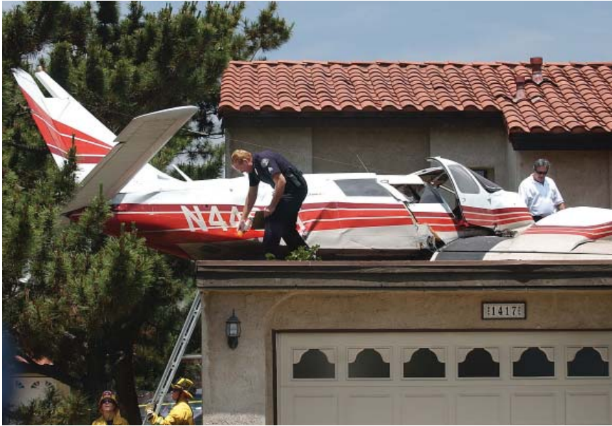
Upland Police Department's Sgt. John Poole and the city's building inspector, Luis Teixeira, investigate the wreckage of a small plane that crashed atop a garage trying to land at Cable Airport, Monday, June 4, 2007, in Upland, California. The crash slightly injured the pilot and two passengers, authorities said. (AP Photo/Inland Valley Daily Bulletin, Mediha Fejzagic DiMartino) (LA Times, Ventura County Star & Riverside Press-Enterprise)
