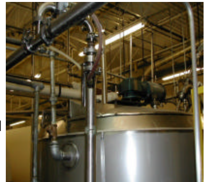
Covered/ventilated flavor tank
