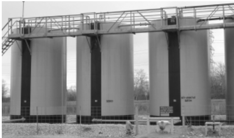
Figure 2. CJ Waller lease water and condensate storage tanks.
