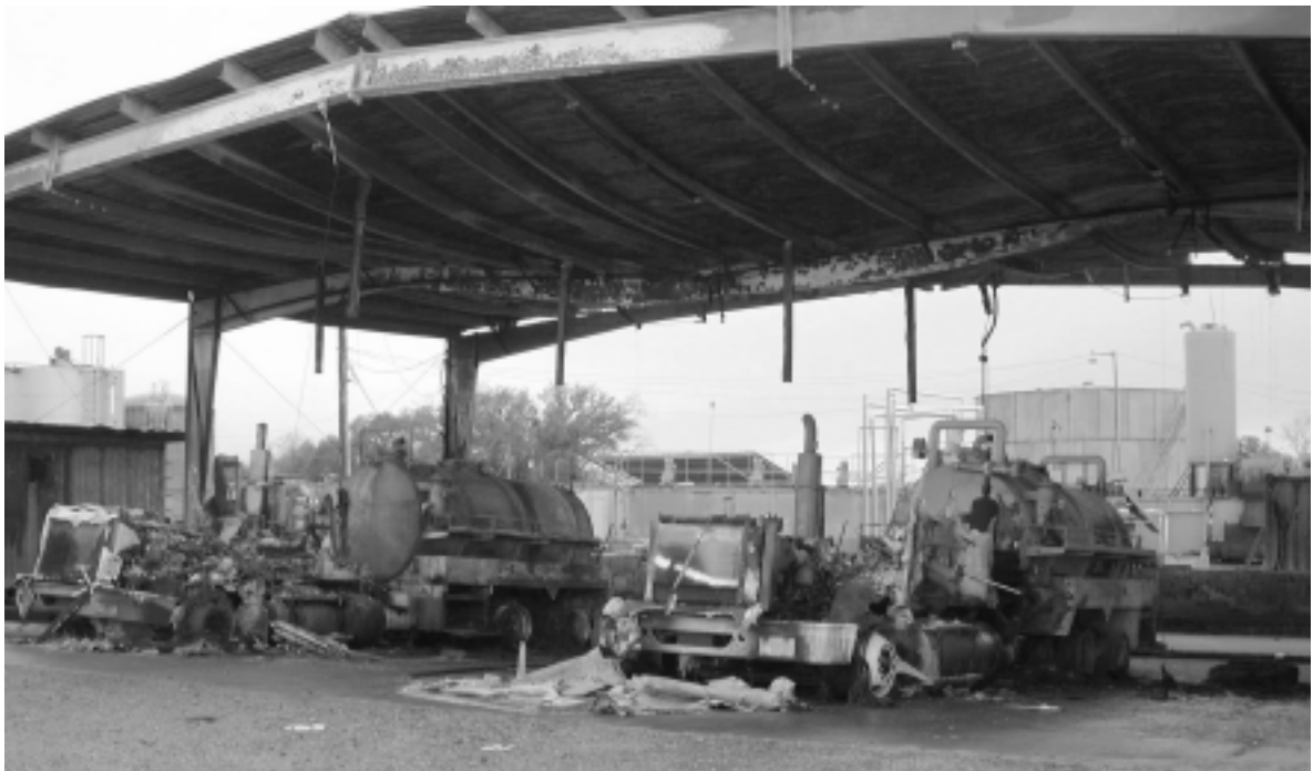
Figure 10. Mud disposal and washout pad, showing burned trucks and damaged canopy.
