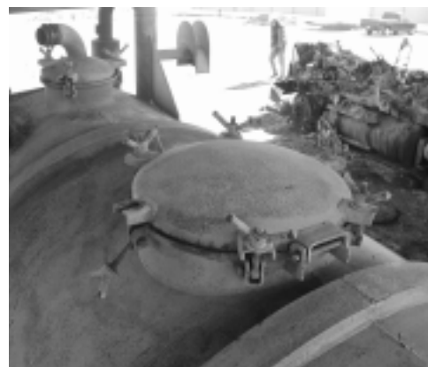
Figure 8. North side truck manway bolts partially removed.
