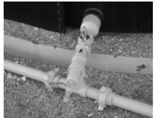
Figure 3. Condensate tank drain manifold and valves.
