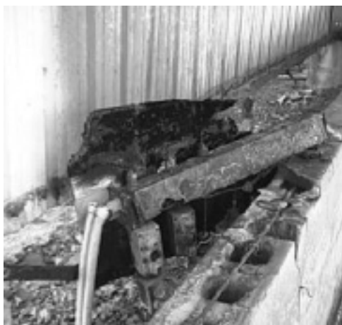
Figure 19. Remains of motor control switch panel.
