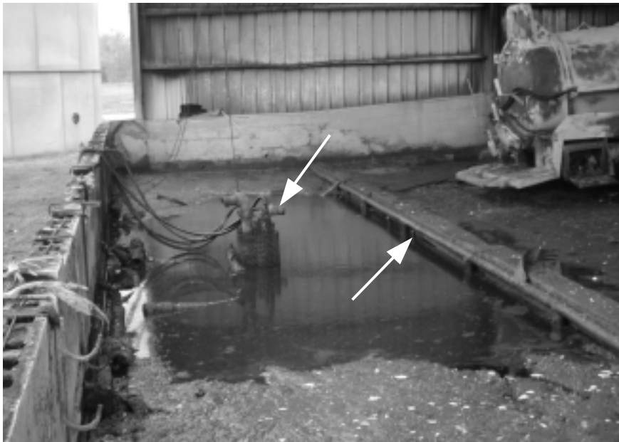
Figure 6. Pad area hydraulic sump pumps and wooden stop beam.
