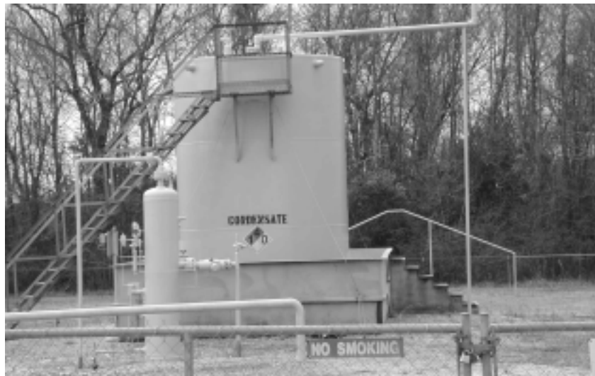
Figure 12. Condensate storage tank located at gas regulator station.
