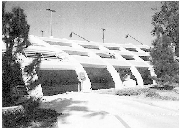
Strong shaking from the Northridge earthquake collapsed this parking structure on the campus of the California State University at Northridge. Because the earthquake occurred at 4:30 a.m., no people were in the structure.
