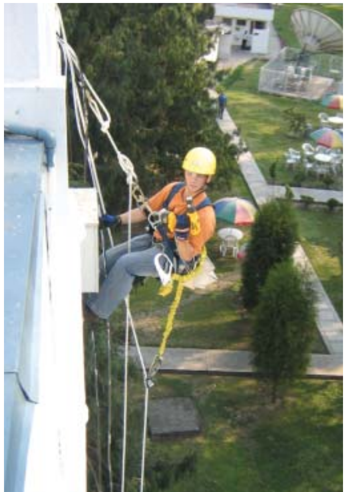
Contractor Brad Raupp uses his rappelling skills during the WEXTEL installation in Kathmandu.
