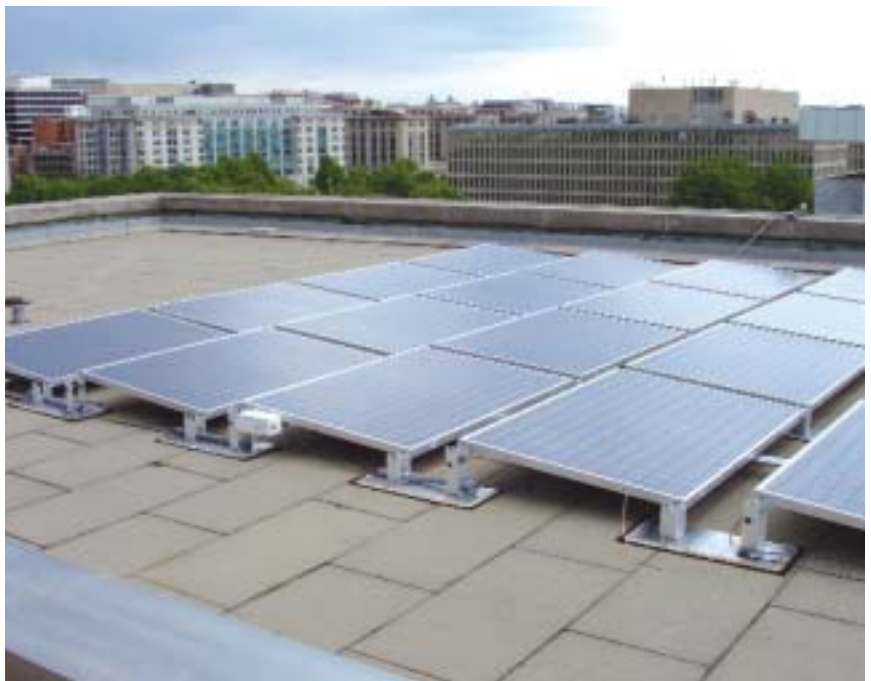
New solar panels grace the roof of the Harry S Truman Building.
