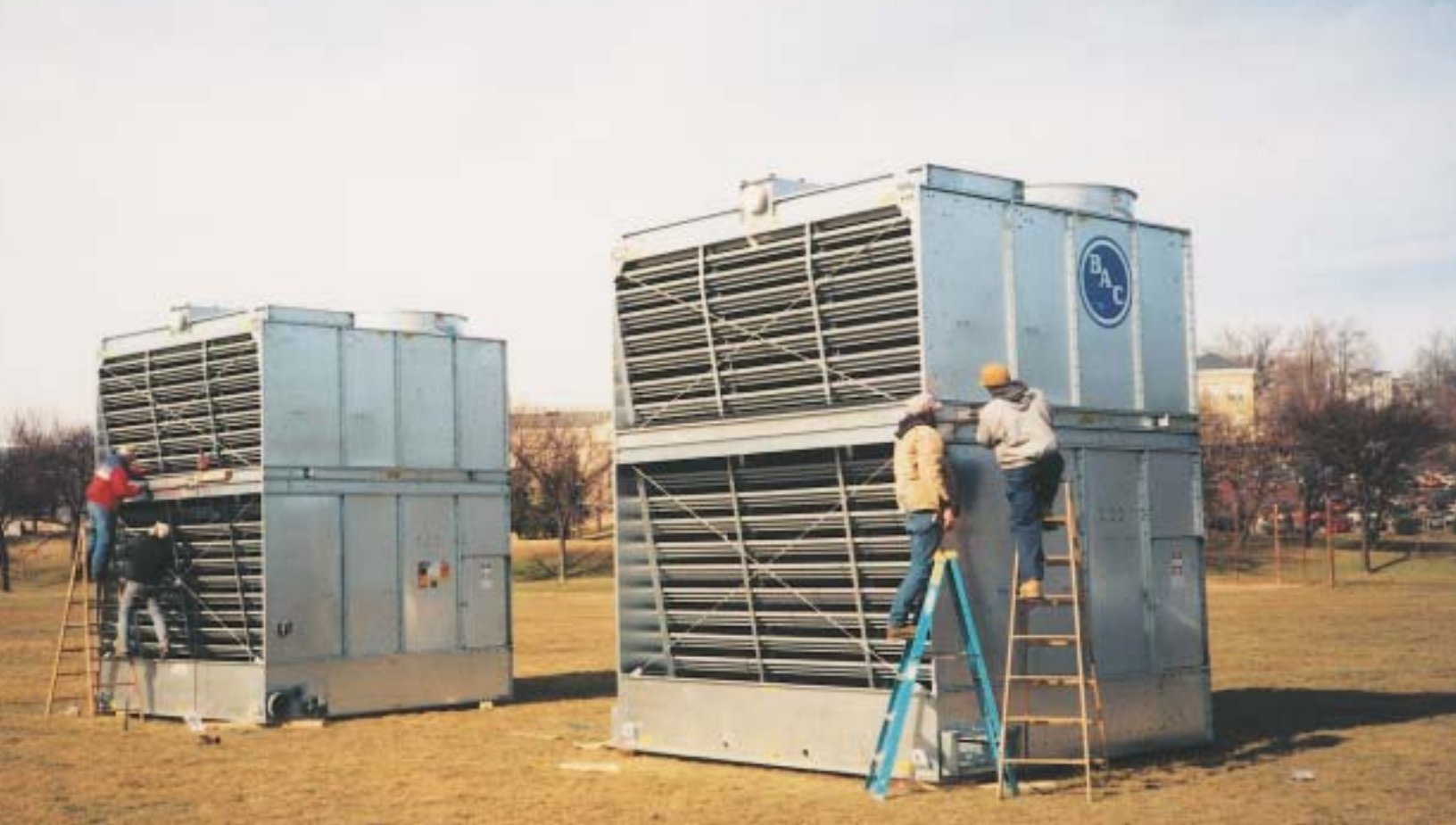
Above, technicians prepare the cooling tower units for the helicopter lift on Jan. 8, 2000. Below, the centralized computer room in State Annex 1. Photo courtesy of GSA
