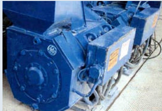
Fig. 8. Electric rig motor
