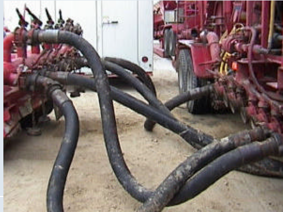
Fig. 8. High pressure lines
