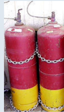
Fig. 4. Properly stored cylinders
