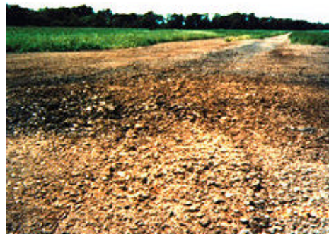
Fig. 1. A plugged and abandoned well site
