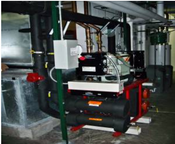
Heat Recovery Chiller
