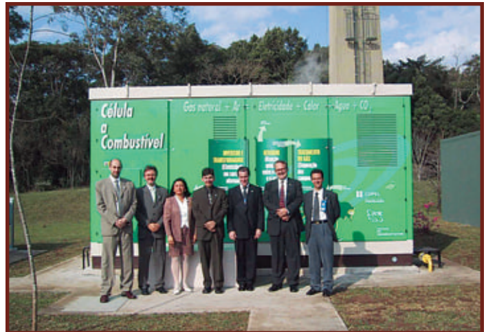
With the help of the U.S. Government, a 200 kw fuel cell is inaugurated in Curitiba, Brazil.
