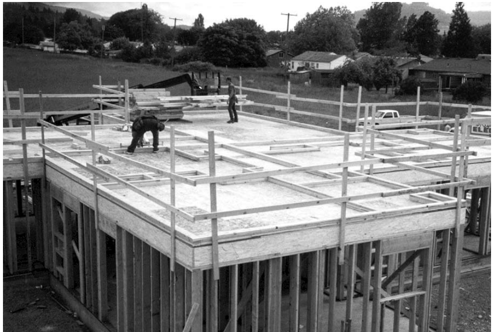
Oregon OSHA Fall Protection — guard rail all around.
