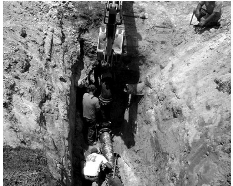
South Carolina OSHA Trenching enforcement action.
