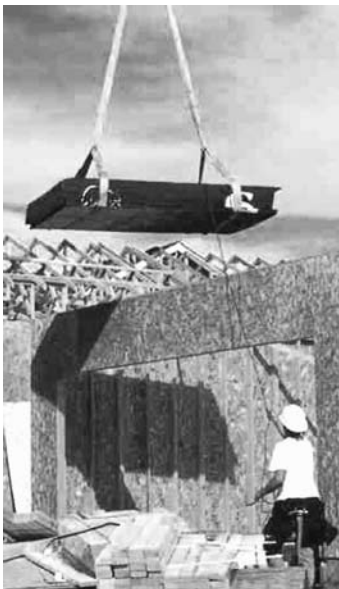
Washington DOSH Crane delivering a sling load. Worker is using a tag line.
