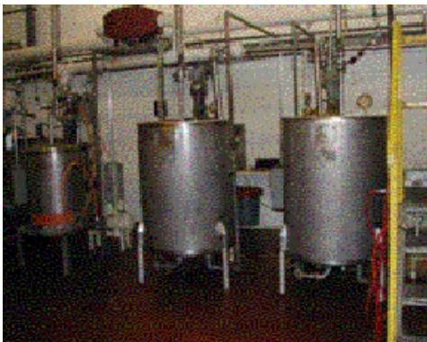
Flavor tank ventilation
