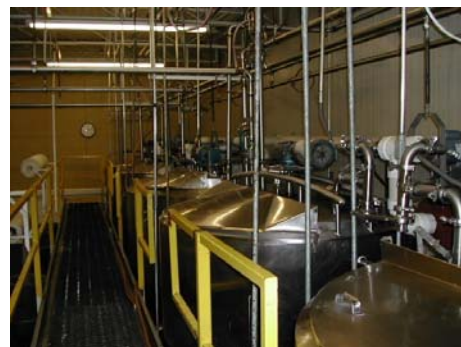
Ventilation of finished oil tanks in mixing room.
