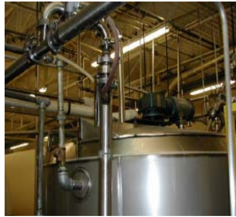
Covered/Ventilated flavor tank ventilation.
