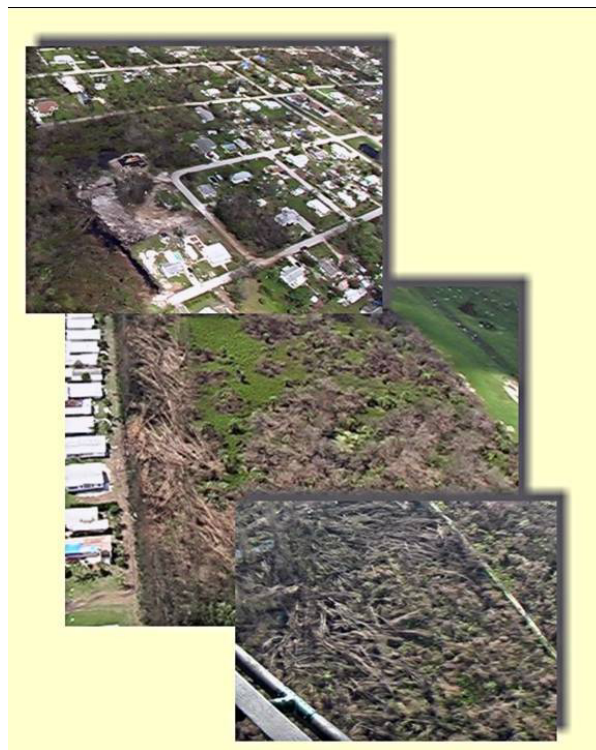
Fig. 13 Photographs of enhanced wind damage associated with Hurricane Jeanne taken from air surveys conducted by the authors. These tornado-like swaths of enhanced damage were observed in extreme Southern Brevard County and occurred as the eye-wall passed over the region. Tree and structural damage within the swaths was much greater than that observed immediately adjacent to the paths.
