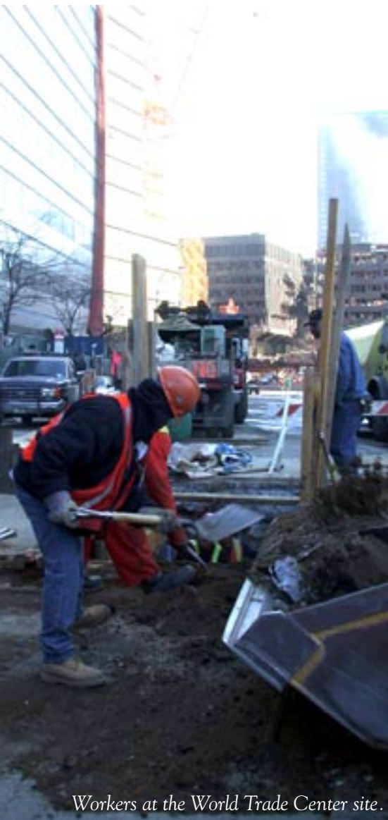
Heavy equipment moves tons of debris from the site. FEMA photo by Michael Rieger
