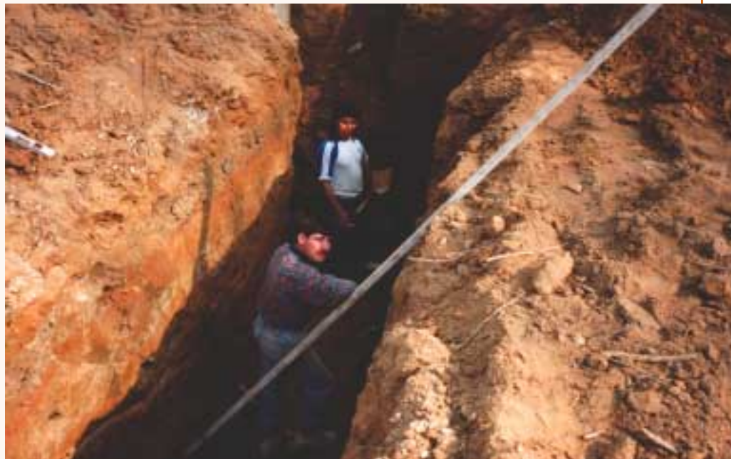
The workers shown here could suffer severe injuries or death from a potential cave-in. The trench has no sloping, shoring, shielding, or safe exit; the workers have no hard hats or personal protective equipment.
