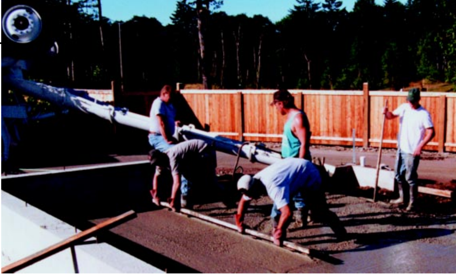
Trainees learn first hand how to lay the foundation for a single-family dwelling.
