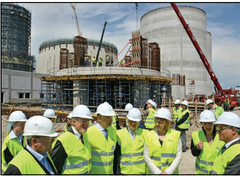
Ambassador Beyrle and local officials learn about the AES Corp. power plant on their tour of the facility, May 2008. [Plamen Ivanov, U.S. Embassy Sofia]
