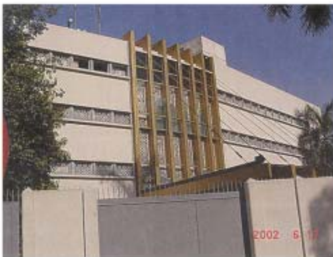
Figure 3: U.S. Consulate, Karachi, Pakistan, after Car Bomb Attack of June 14, 2002, Showing Little Damage to the Building
