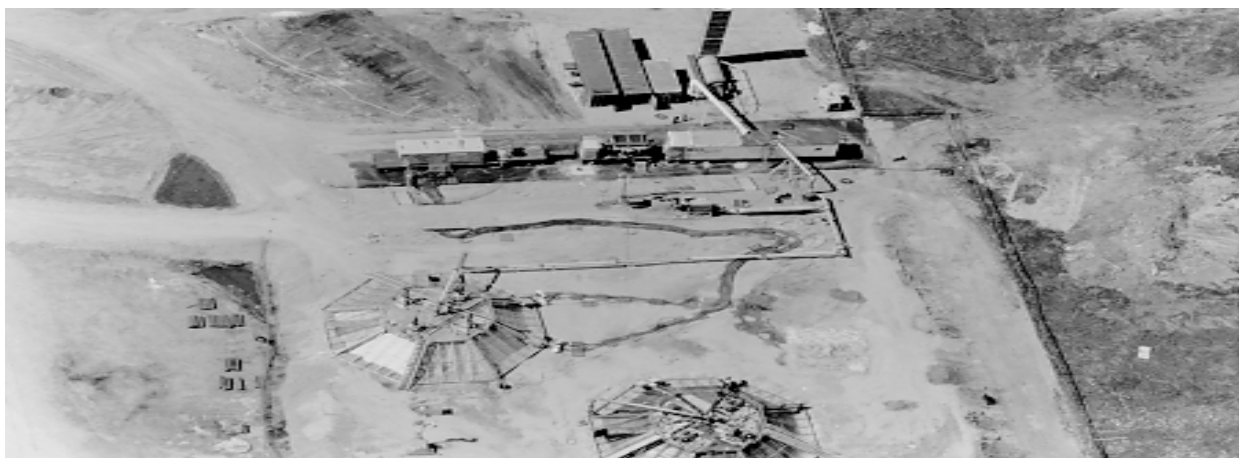
In Situ Vitrification Process Equipment
